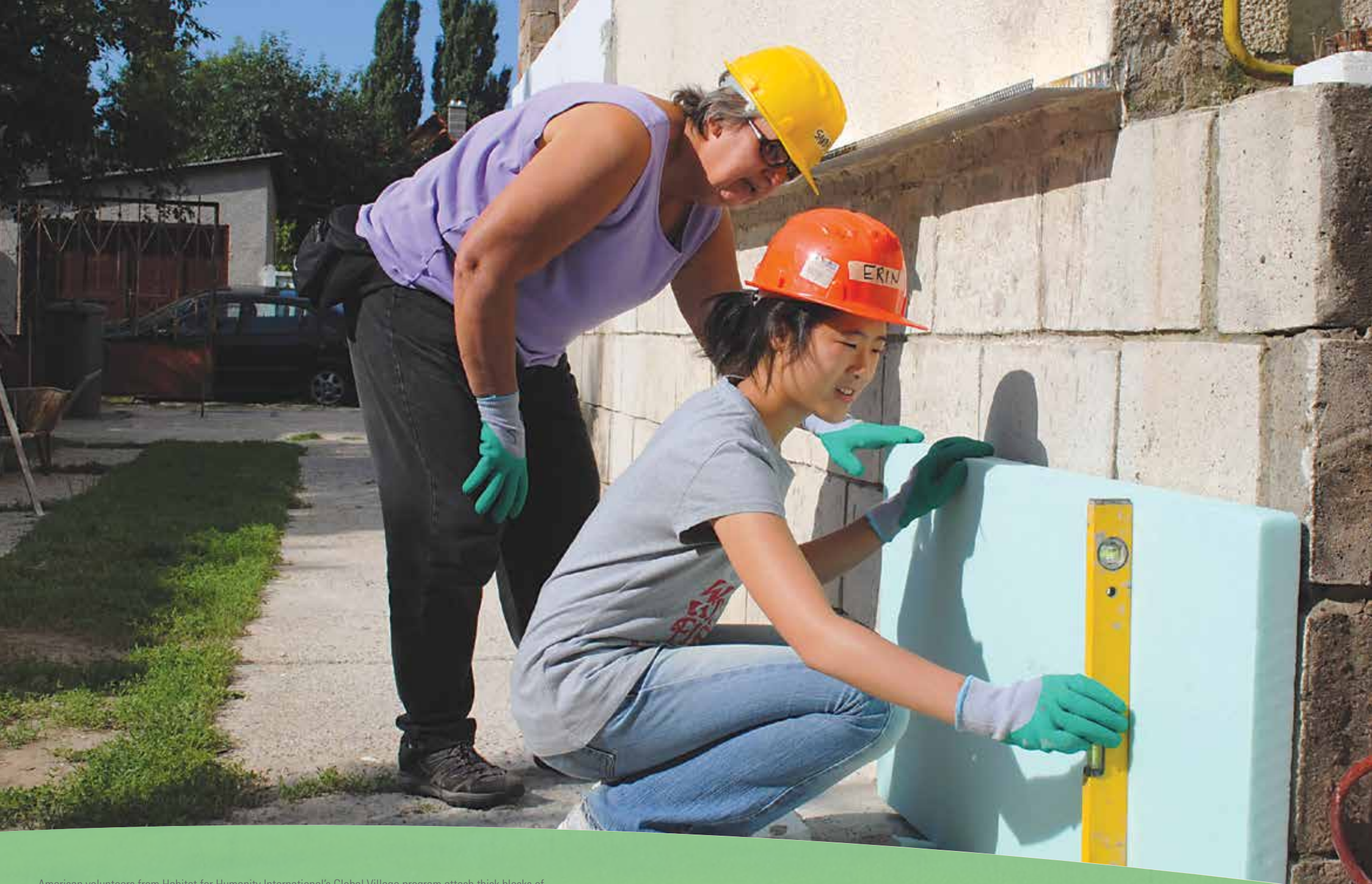
American volunteers from Habitat for Humanity International's Global Village program attach thick blocks of insulation to the exterior walls of a house in a small town north of Budapest, Hungary.
