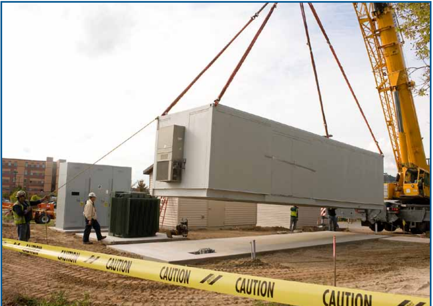
The U.S. Department of Energy's Midwest Clean Energy Application Center at the University of Illinois at Chicago's Energy Resources Center provided technical assistance to Gundersen Lutheran Health Systems to determine the initial feasibility of the landfill gas combined heat and power plant being installed on the health system's campus in Onalaska, Wisconsin.
