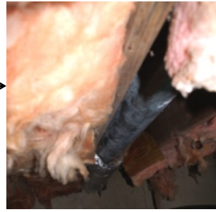
Uninsulated Ducts in Crawl Space
