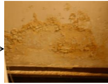
Mold on Walls
