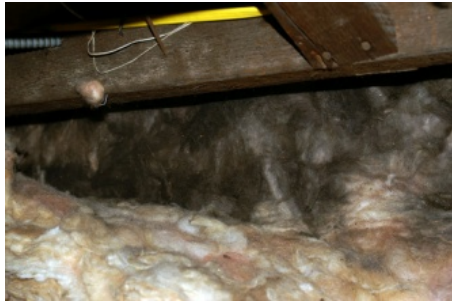
Unsealed Rim Joists
