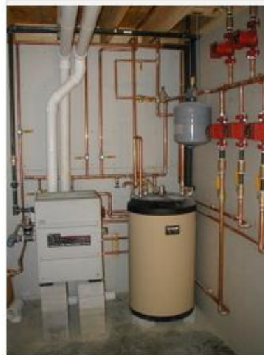
High-efficiency boiler with domestic hot water tank.
